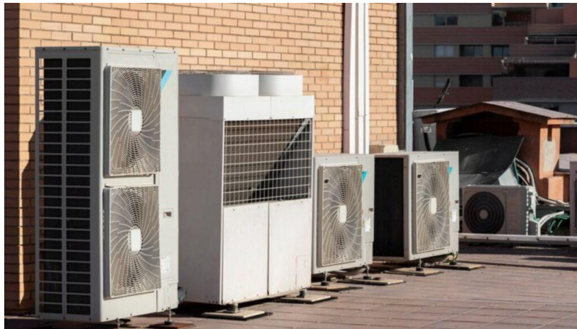
Figure 24. Air Source Heat Pump
