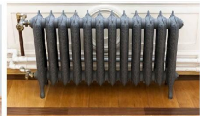
CAST IRON RADIATOR
